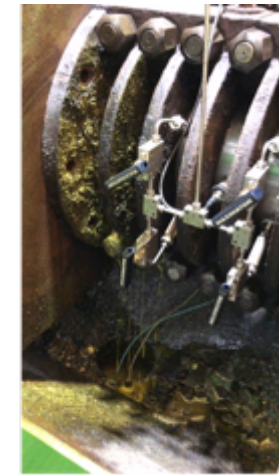
CO 2 injection into strainer
